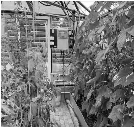
Fig. 3. «Rozumnytsia» greenhouse automation complex
