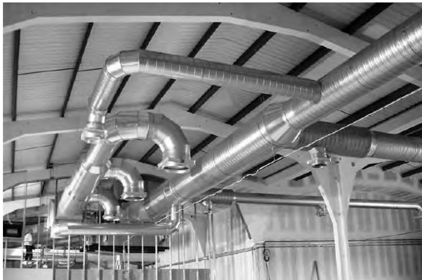
Fig. 1. Ventilation system in the production premise
