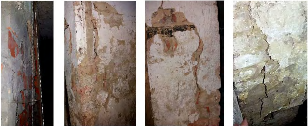
Fig. 3. Visible loss of resistance, as well as vertical and horizontal cracks in the middle bearing wall on axis B in axes 6–8
