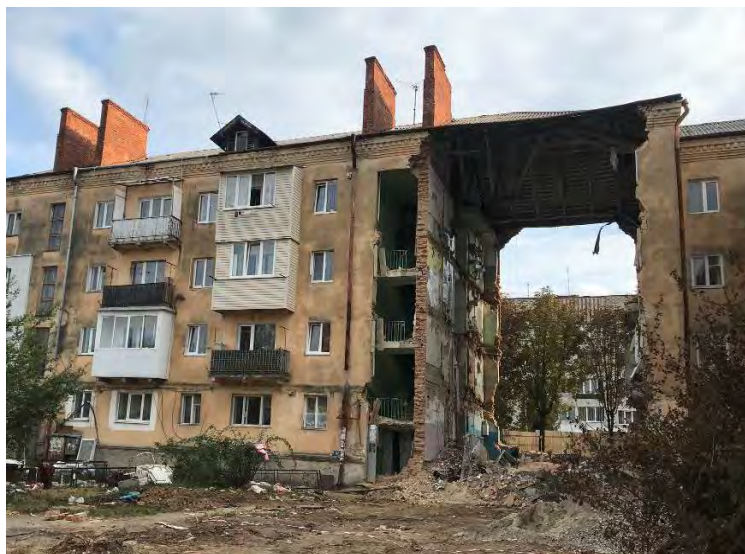
Fig. 2. The collapse of part of the building
