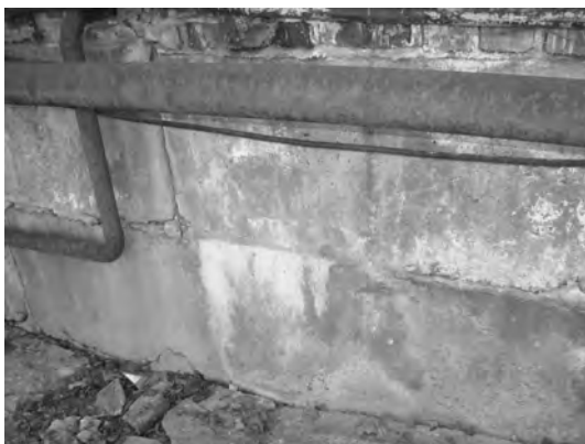
Photo 3. The state of the foundation of wall blocks by axis "B" between axes "1/1" ... "3". Moving units by horizontal and vertical seams and by contact of walls and blocks
