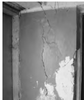
Photo 7. Vertical crack of the wall on the first floor along axis "2" between axis "A"... "B"
