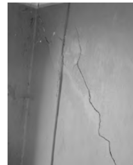
Photo 8. Vertical crack of the wall on the second floor at the crossing of axis "A"... "1/1"
