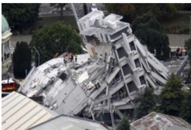
Fig. 1. Importance of safety factors: collapse of a 5-storey RC building in Christchurch (New Zealand) after the 22 February 2011 earthquake
