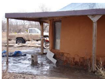
Pic. 8. A low base and a slope from the house can be disastrous when spring flood or abnormal rainfall.
