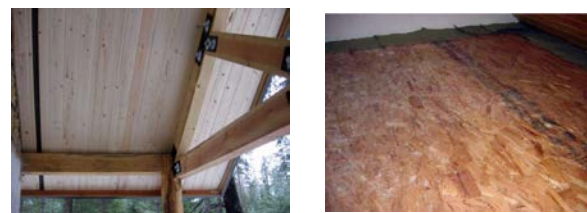
Pic. 28. Ceilings and a roof in the house of straw are sheathed with lining
