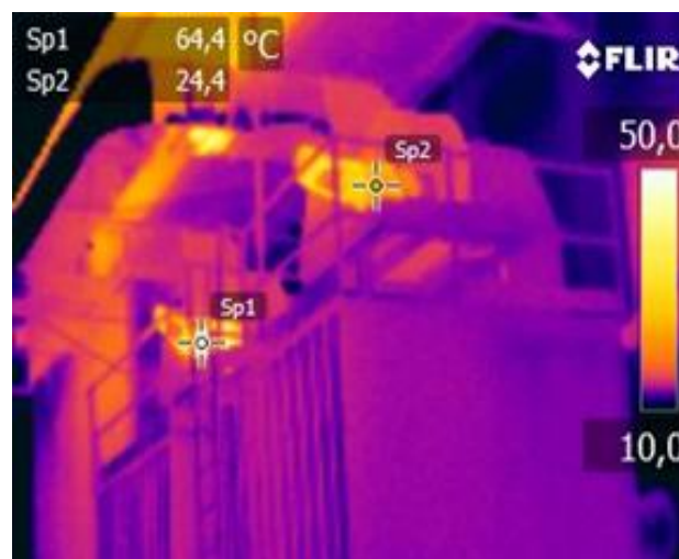
Fig. 1. Thermography of a ventilation system. The two electric motors are the same size and the same nominal load but the surface temperatures are very different: a warning sign of possible energy waste
