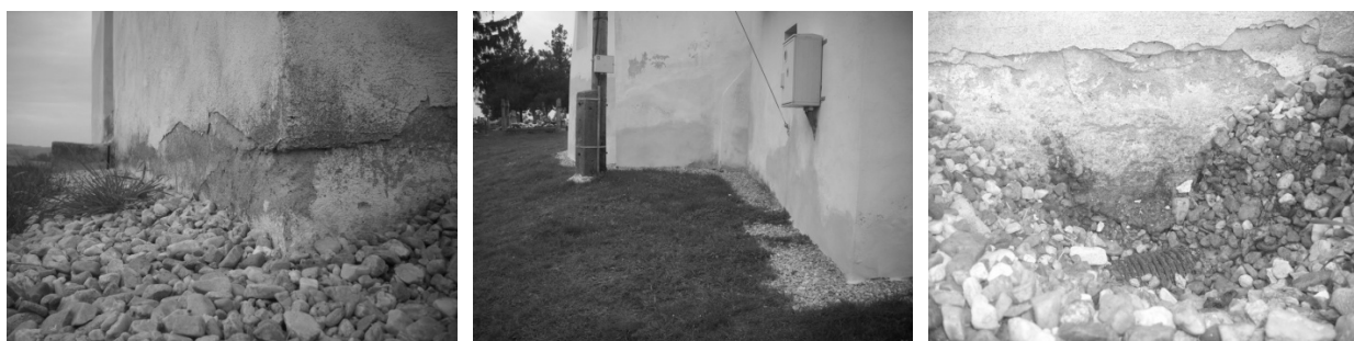
Fig. 3. Damages on the church Gemersky Jablonec: 1 – damp on the facade; 2 – damp maps on the wall; 3 – nonfunctional drainage system
