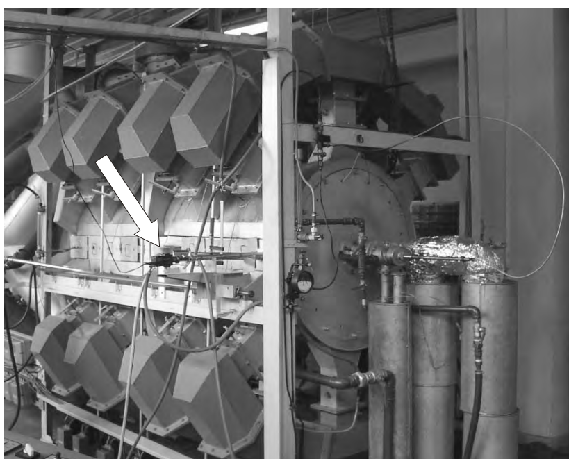
Fig. 1. Combustion chamber at Institute of Power Engineering. CCD camera mounting is depicted with an arrow
