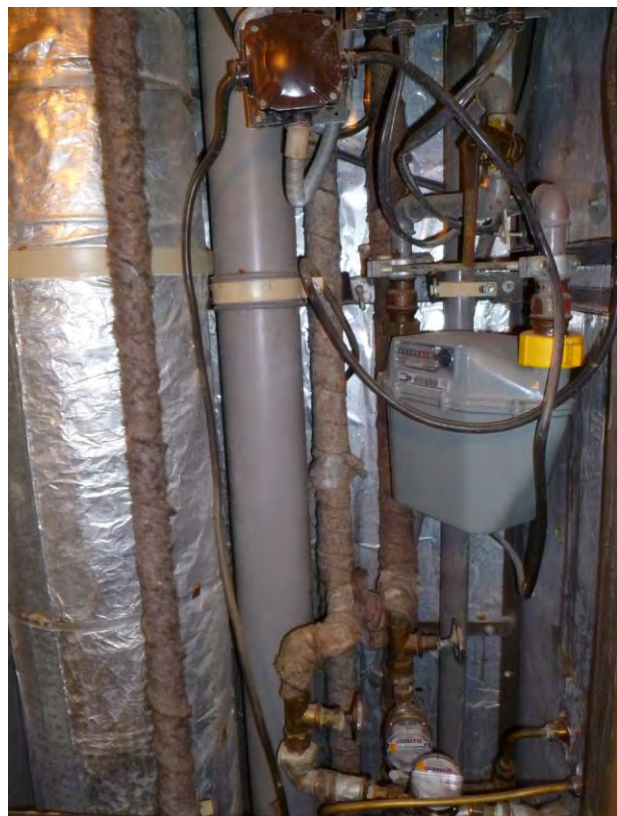
Fig. 2. The view on origin distribution pipes
