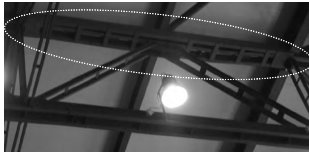
Fig. 9. The strengthened top chord of the truss tie-beam (in the area over the fire)
