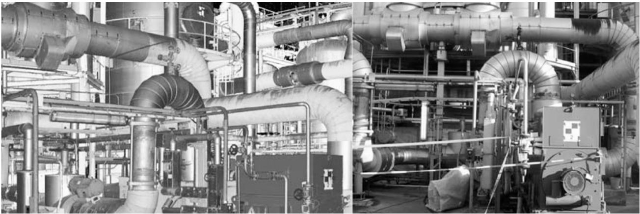
Fig. 4. Intensity image (left) vs. colour image (right) for an industrial plant (by Przybilla 2005)
