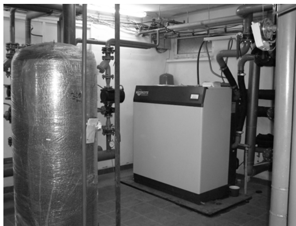
Figure 2. Heat pump in the boiler room
