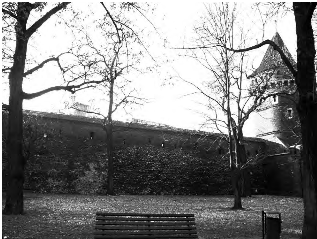
Fig. 11. Western curtain wall from the north, pre-conservation condition, photo by. E. Wyszynska.
